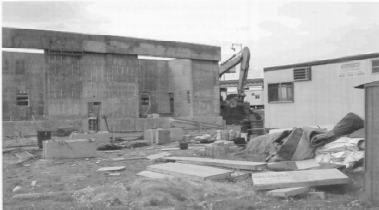
A view of the new Dechlorination Facility which is being constructed by Scuffor Construction of Newark, New Jersey. This building is located at the west side of the aeration basins. This facility is necessary to meet the N.J. Pollution Discharge Elimination System permit. It will remove chlorine from the plant effluent. It is expected to be completed by the end of 2000.
